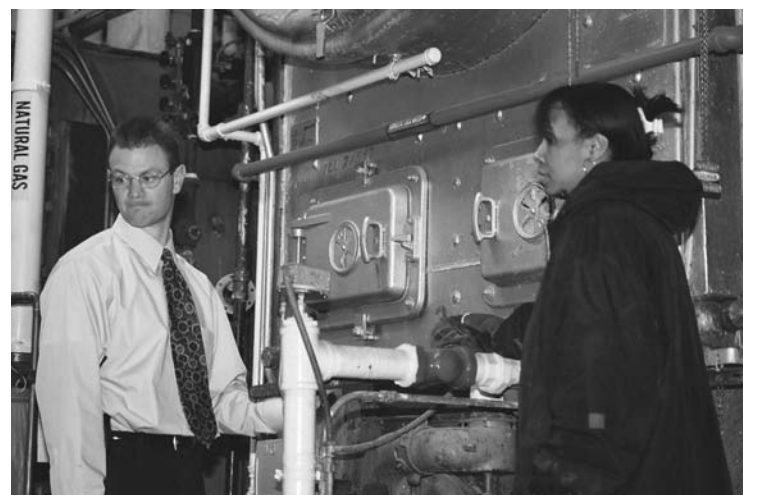
Assistant Principal Ken Bonomo and Head Custodian Tria Akines look over one of the school's three boilers, which need repairs as often as three times a week.
